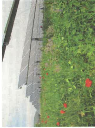
Saint-Restitut (26) - Structure trackers
